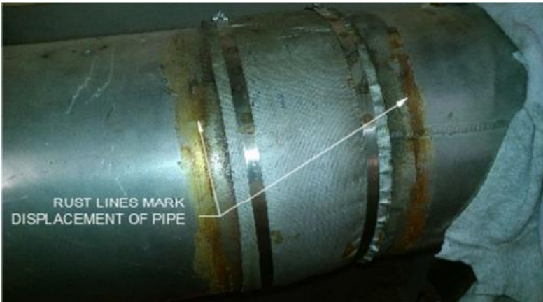
Photo illustrating the movement of pipe at flexible connector piece.
