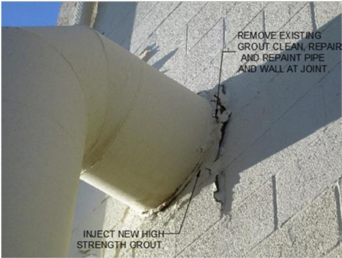
Photo of the damage done to the wall due to movement of the east pipe, along with recommended repairs.
