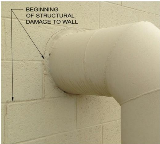
Picture illustrating beginning of damage to wall around west pipe.
