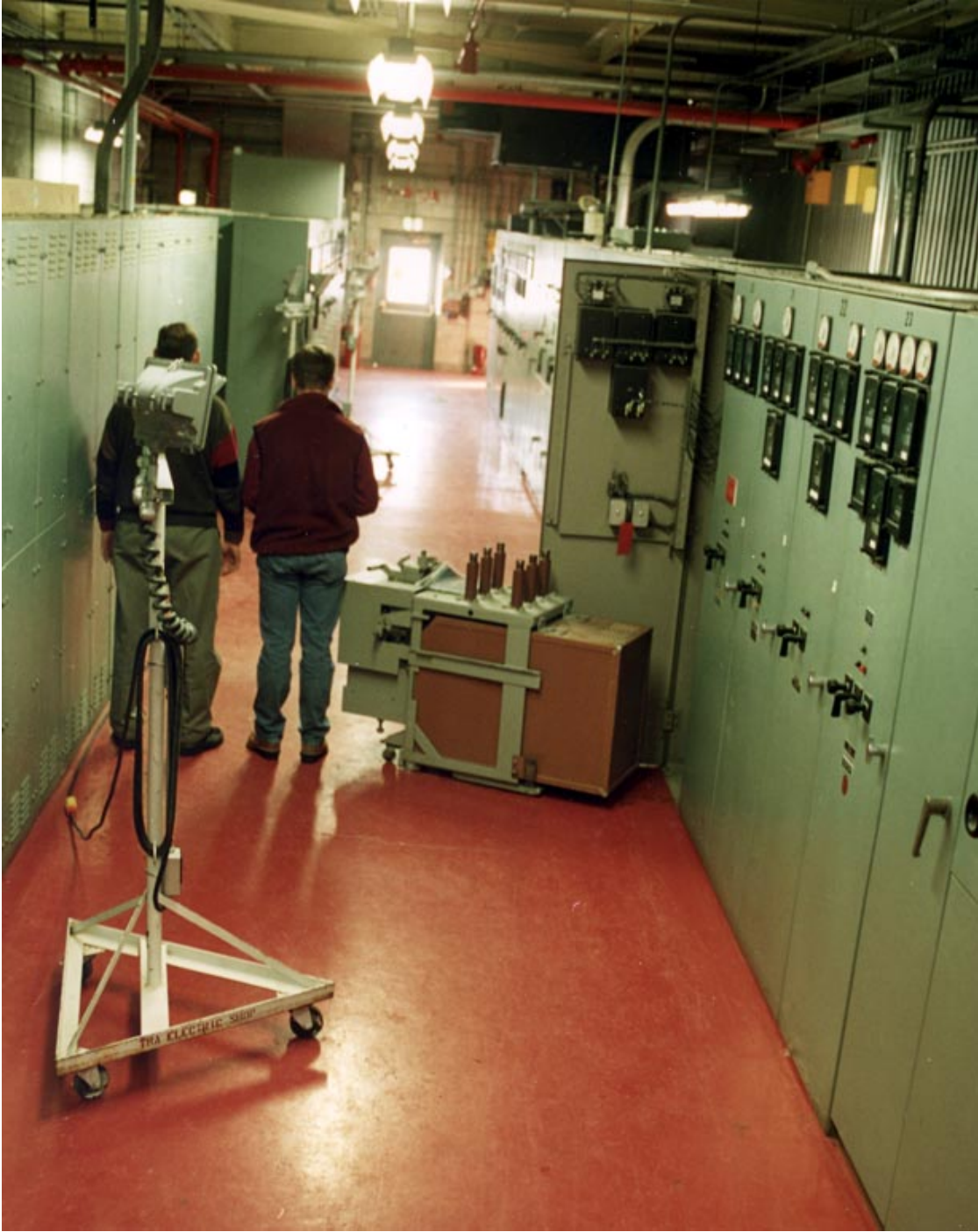
Figure 2-1. Clear egress path around electrical work equipment.
