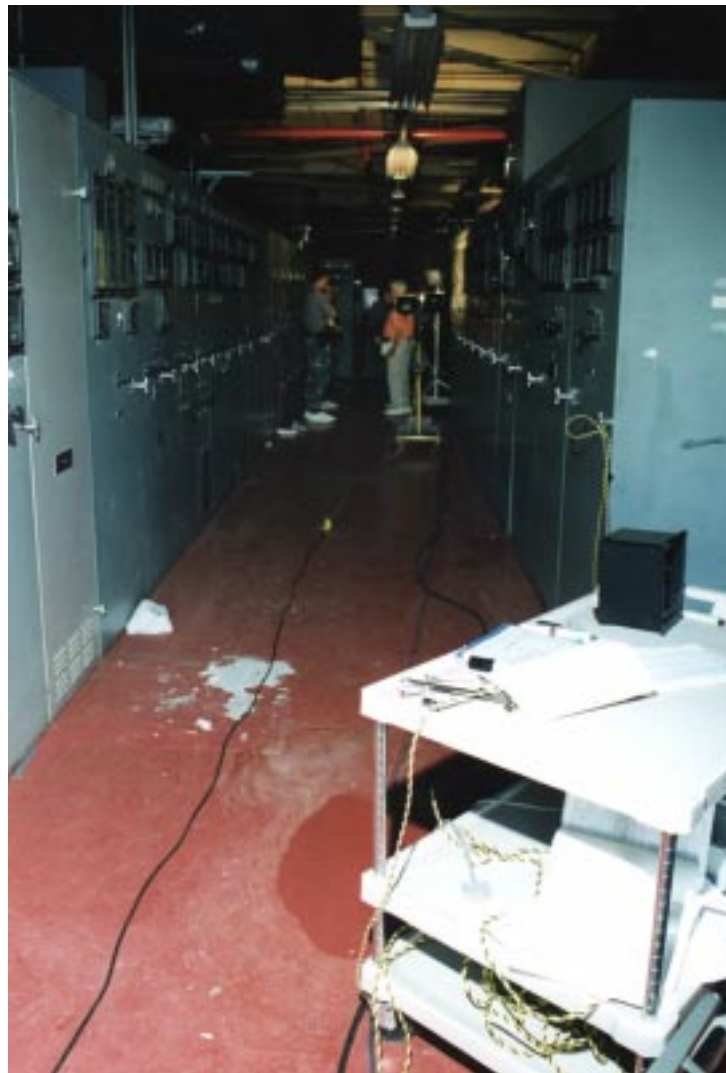
Figure 2-2. Clear egress path to west door remains even after equipment was moved during the rescue.
