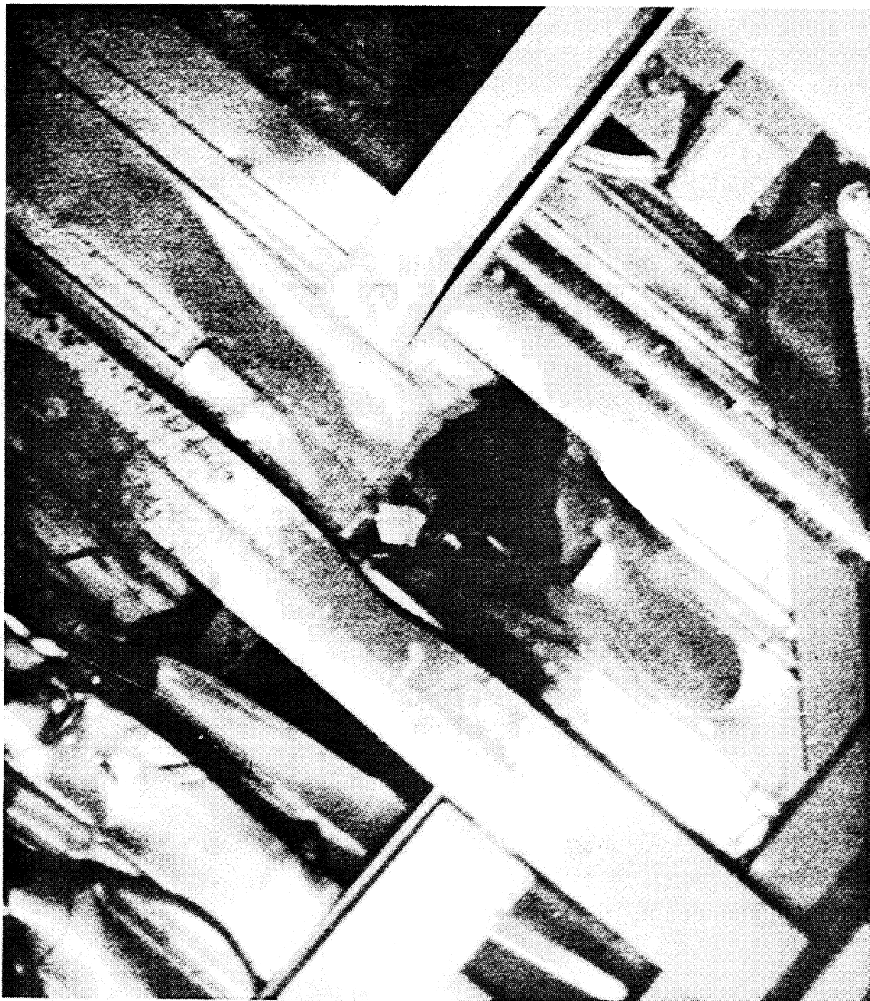
DAMAGE TO FAN FLOOR ABOVE REACTOR HEAD
