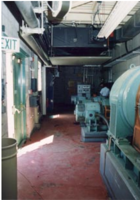
Exhibit 2-3. Motor Generator Room Near South Door
