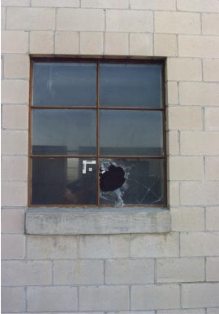
Exhibit 2-4. Broken Window, South Side
