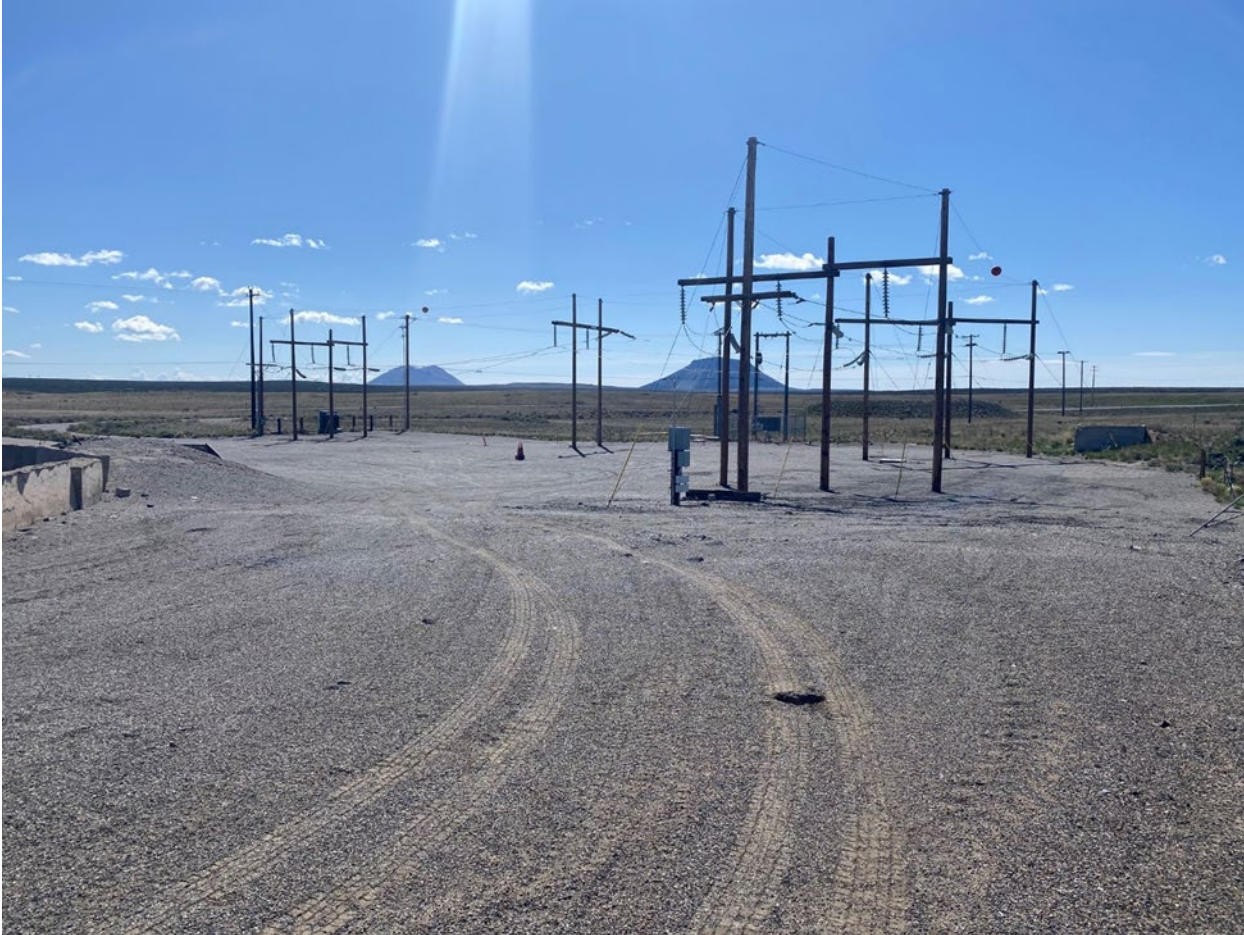
Figure 1. Existing Electrical Structures.
