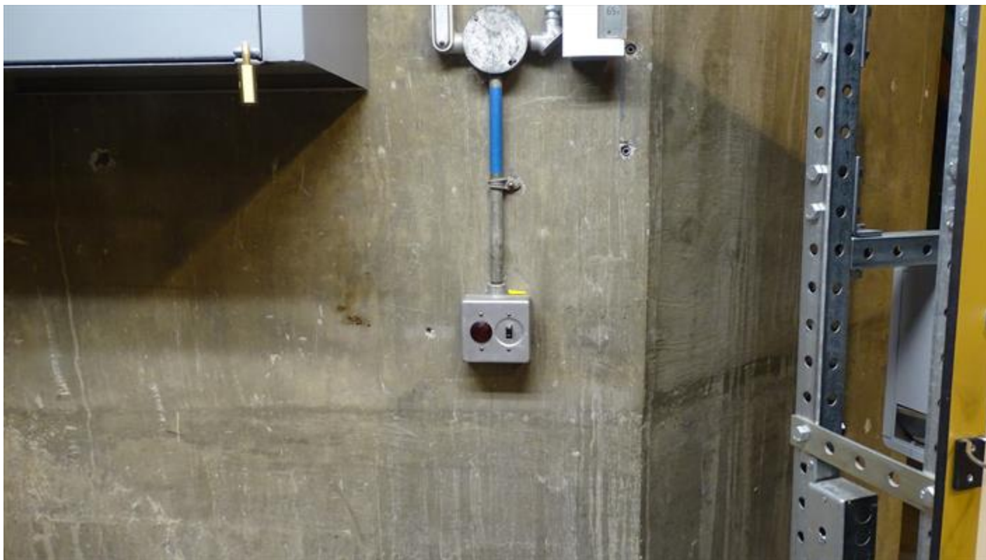
Figure 8. Light switch with burned out indicator.
