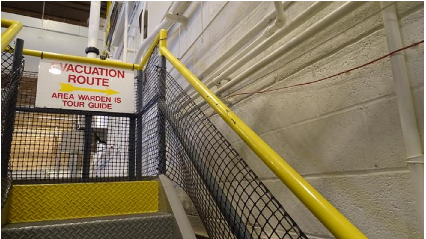
Figure 5. Stair in northwest corner of low bay, showing paint loss.
