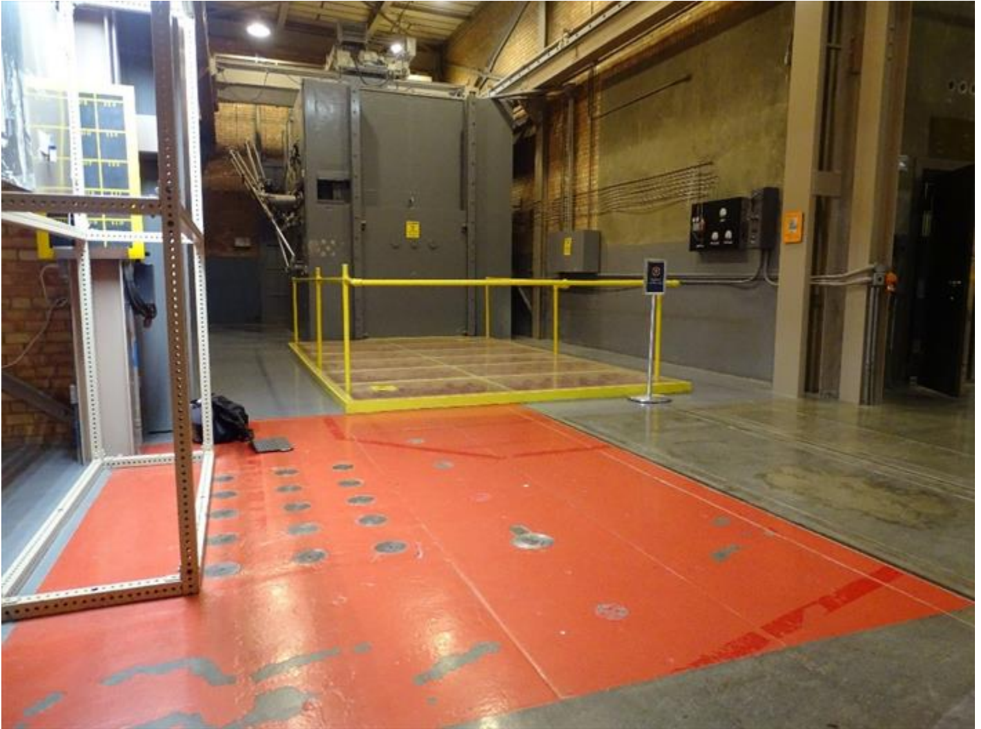
Figure 9. Area over Wash Room showing paint loss.
