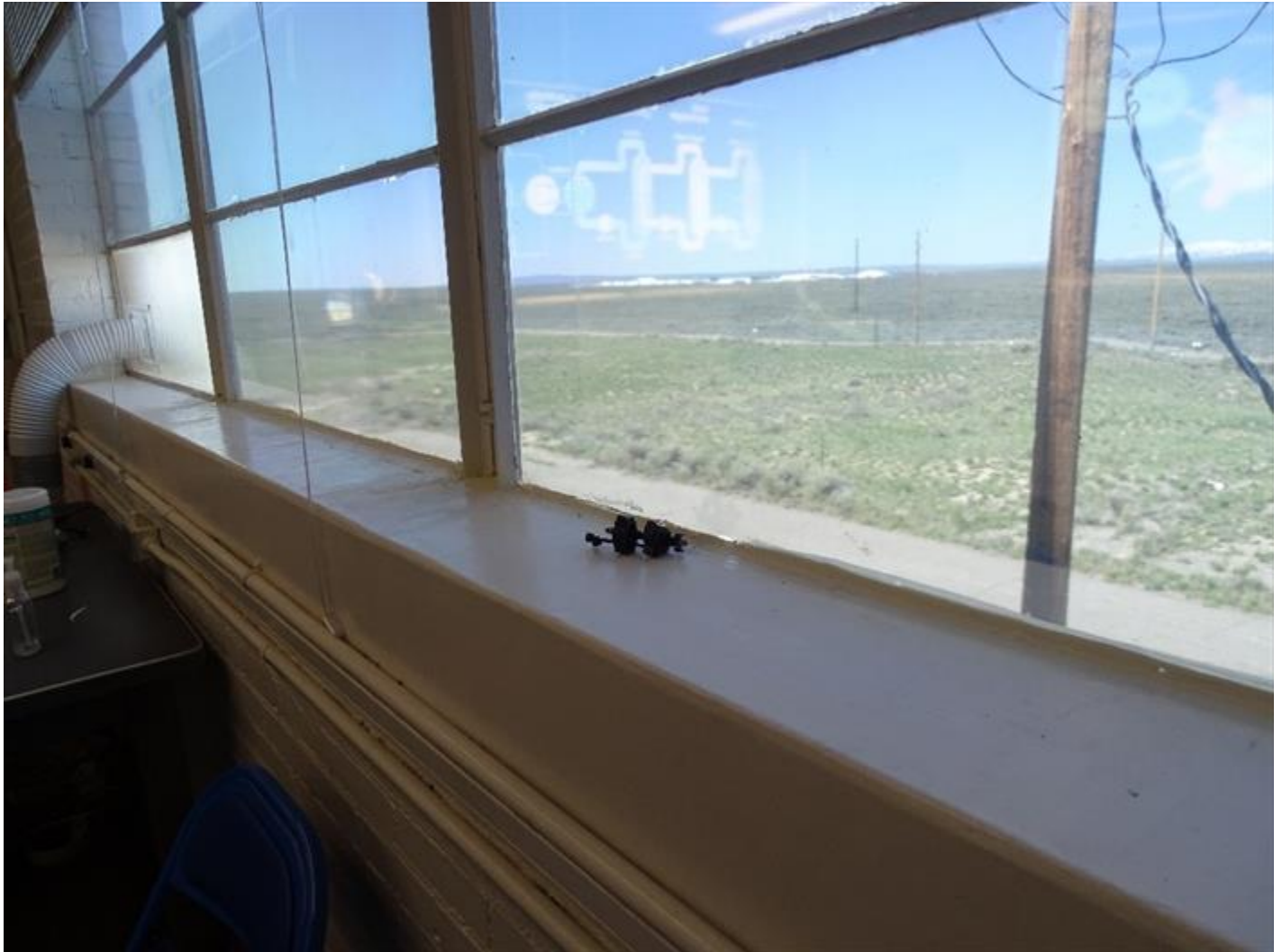
Figure 2. Windows in classroom with failing UV film.
