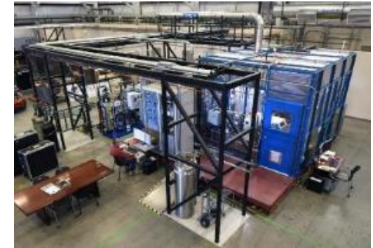
25 kW high-temperature electrolysis @ INL Energy Systems Laboratory
