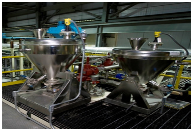
An interior feed skid located within the Integrated Waste Treatment Unit
