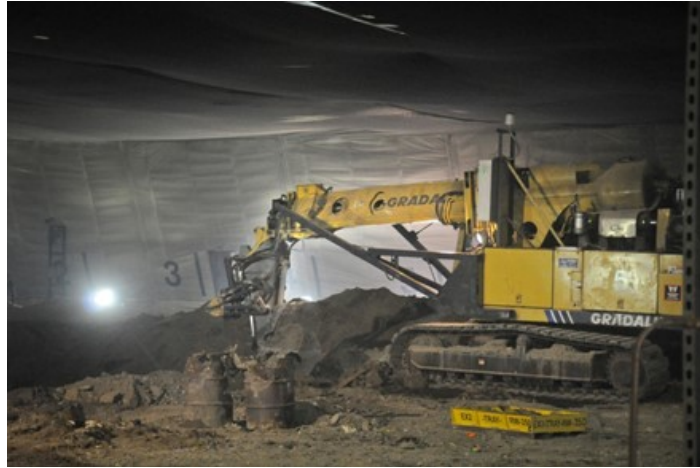
A specially modified waste excavator was used to remove transuranic waste from Pit 9.
