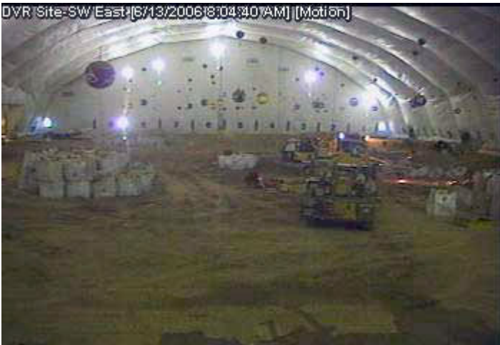
After the initial Pit 9 failure, meanwhile, The current approach to buried waste retrieval involves using specially-fitted backhoes inside temporary containment facilities to dig up the targeted waste
