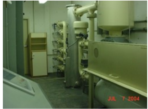
This unit is one of several that is used to "vacuum" volatile organic contaminants from the zone beneath the buried waste, removing them before they migrate into the Snake River Plain Aquifer below.
