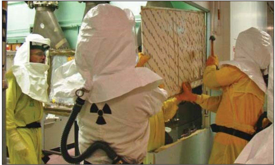
Workers remove a section of a wall in the former Analytical Laboratory at Hanford's Plutonium Finishing Plant. The work is part of the ongoing decommissioning of the complex.
