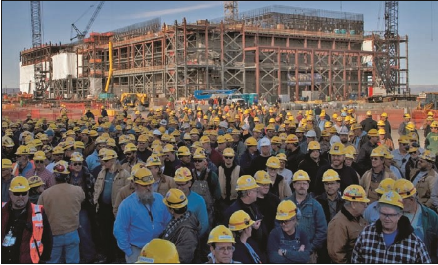
Workers gathered in front of the Pretreatment Facility that is part of the Waste Treatment and Immobilization Plant at the Hanford Site to celebrate reaching the 50 percent complete mark on the overall project.
