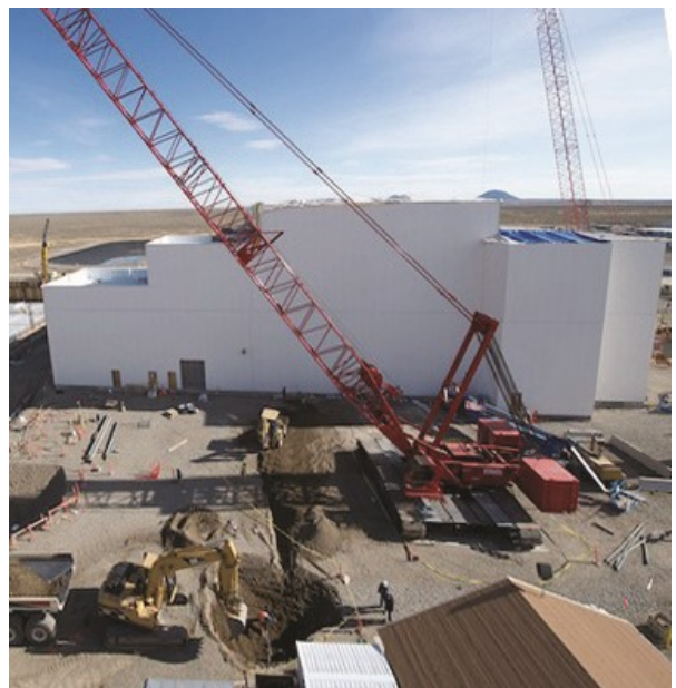
With the walls and roof now in place, construction on the Integrated Waste Treatment Unit at the Idaho Site can continue through the winter months.
