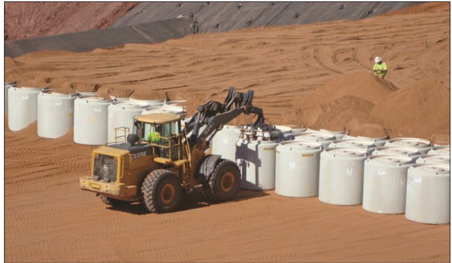
The last of the Fernald waste canisters being placed at the Waste Control Specialists facility in western Texas.
