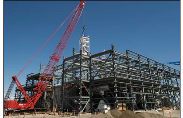
The largest of six process vessels for Idaho's Integrated Waste Treatment Unit being hoisted into place on September 2.
