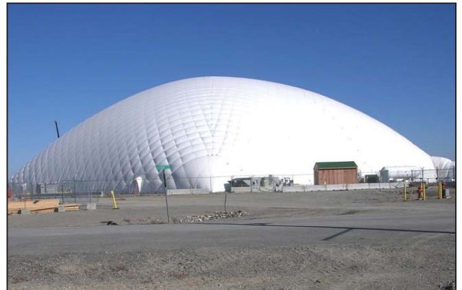
This inflatable heated tent sheltered work on the IWTU through two winters before it was taken down in April.
