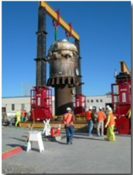
ETR vessel removed from substructure. Vessel lifted approximately 40 ft. - Click on image to enlarge.
